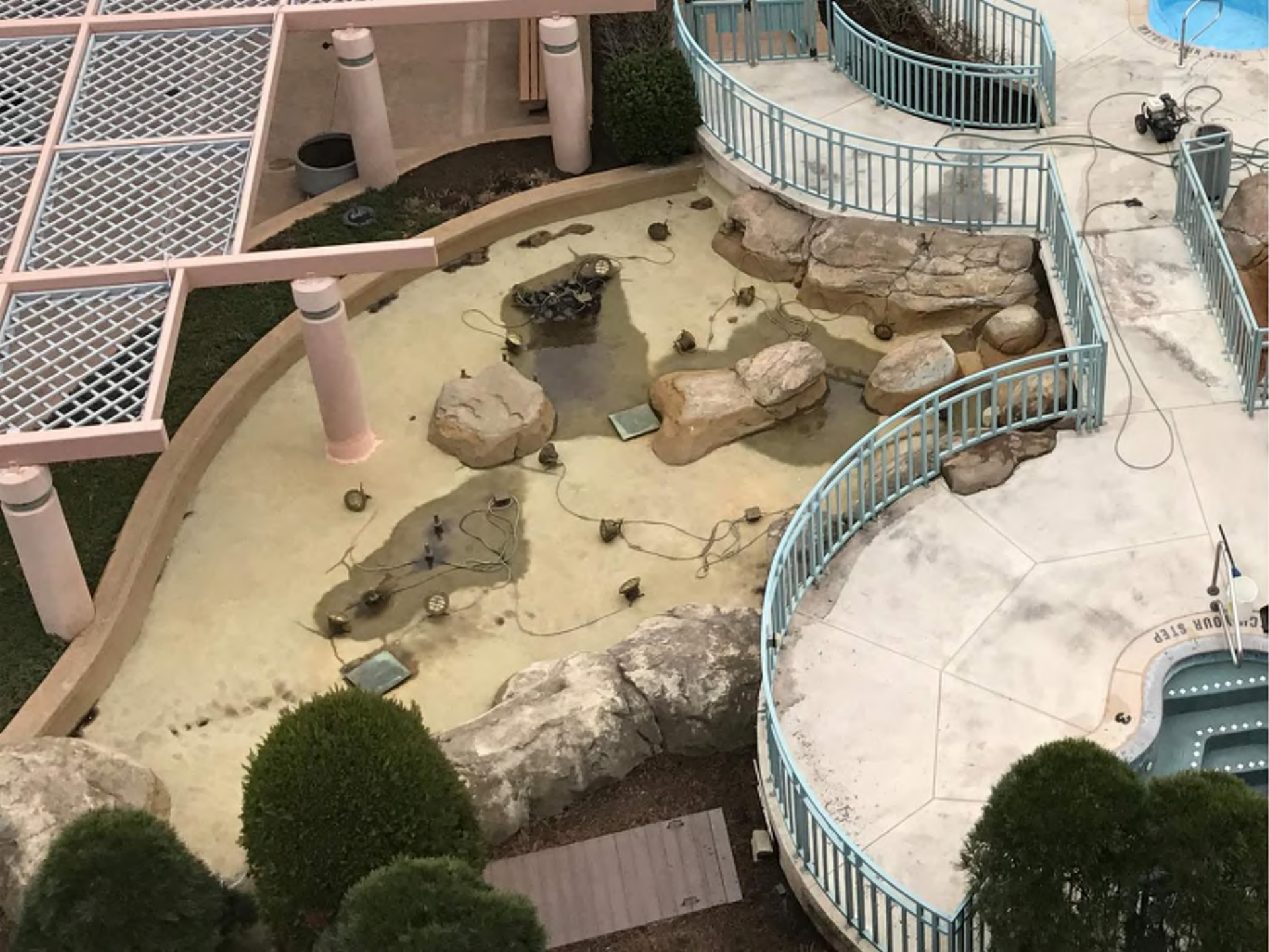
DETERIORATED LAGOON AREA
